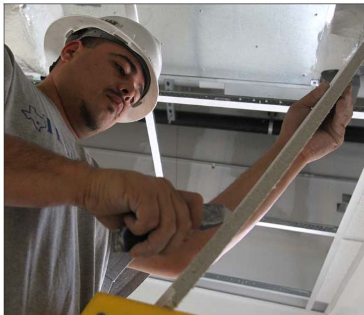
A Tejas Premier worker installs ceiling tiles in the building. Carielo said, "Now, about 60 percent of my work is going to be federal projects."
